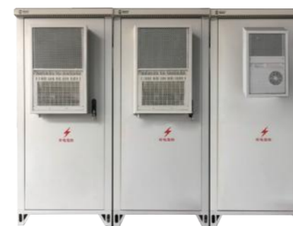
三柜/Three cabinets 380Vac/48Vdc/600A/400Ah Three Cabinets
